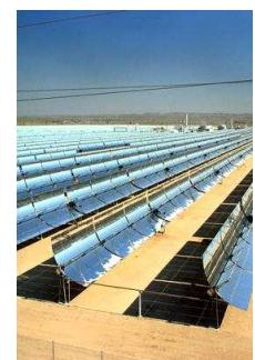
A Solar Photovoltaic (PV) array
